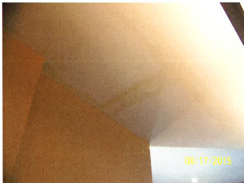
Room 206 wet south wall and water stained ceiling
