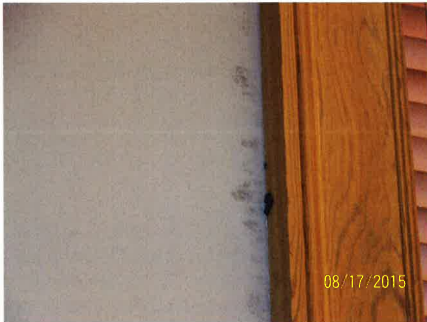
Room 303A wet south wall and visible mold along window frame.
